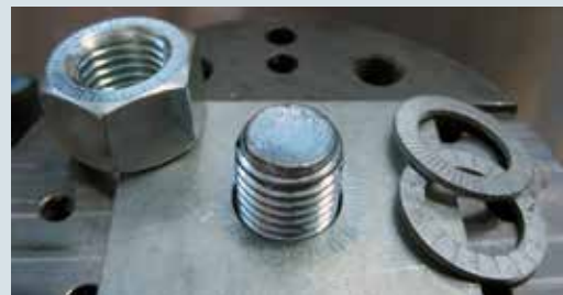
After disassembly, impression marks must be visible on both the fastener and the contact surface.
